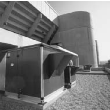
Air conditioning application
